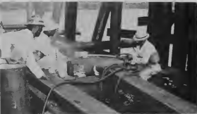
AIR-DRIVEN chain saws speeded pipe trestle construction. CADENA movi cu aire ta zaag construction mas liher.
